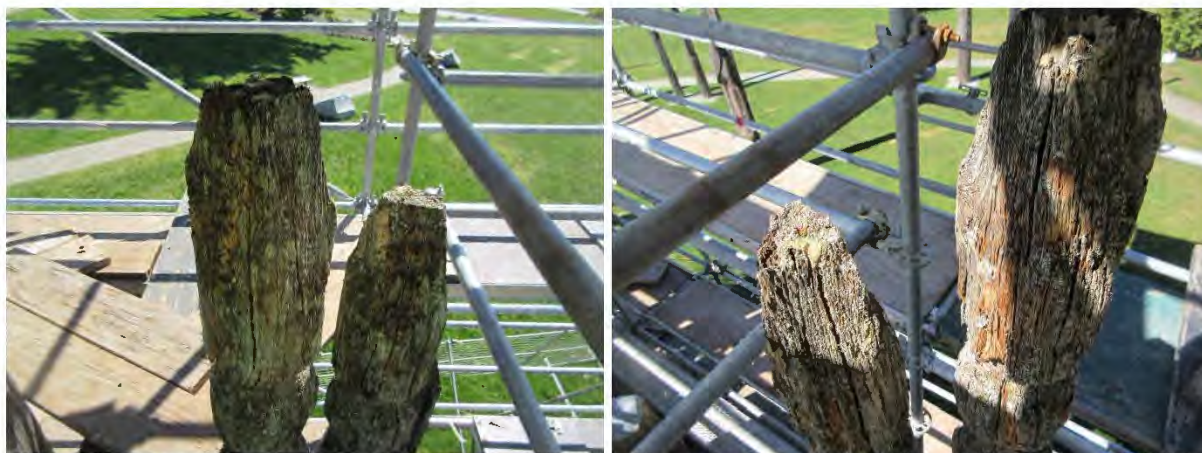
Unit #1, detail of “The Gods and the People”. Note conditions of exfoliation of surface wood grain and surface weathering.
