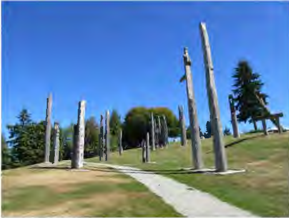
The totem poles on the lower slope of the hillside are on flatter ground and are a concern for moisture retention and subsequent fungal rot of wood at ground level.
