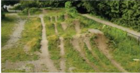
Example of jumps eroding.
