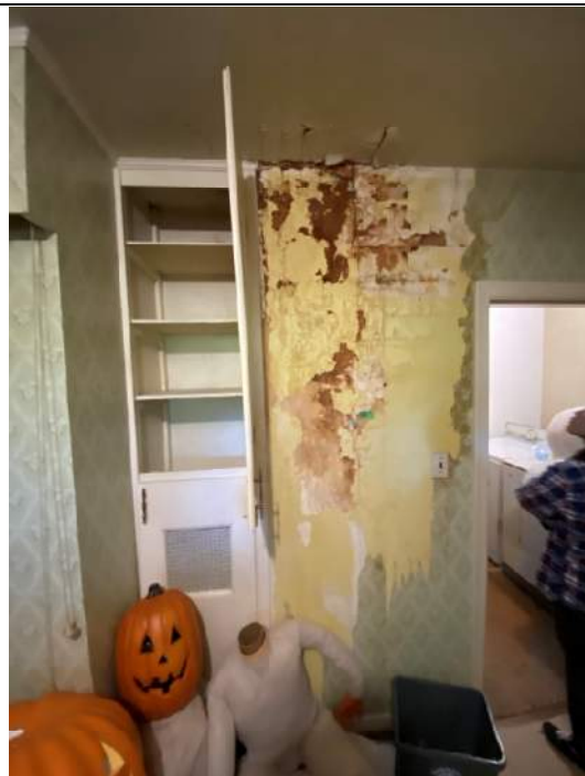
Figure 20: Bed Room, showing water leak.
