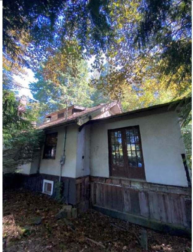
Figure 5: 2023 west elevation. Rear yard, including the addition (sunroom) with the missing patio.
