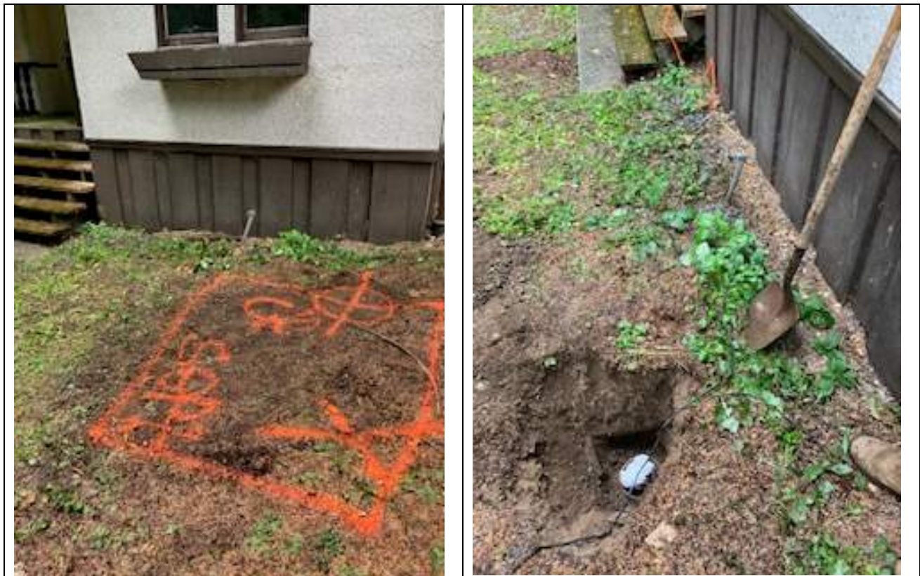
Figures 11 & 12 – Location of the existing Septic Tank in front of Hill Cottage (east elevation).
