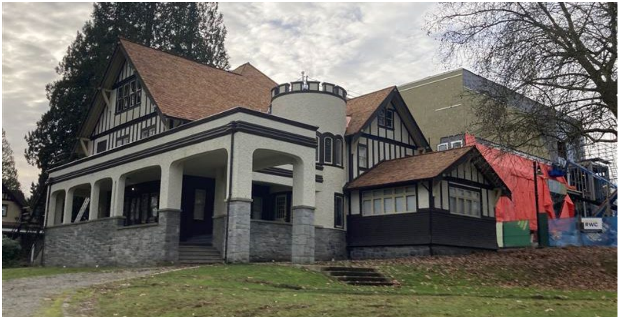
The W.J. Mathers house with its new cedar roof. The chimneys have been temporarily dismantled above the roofline due to concerns about their stability.
